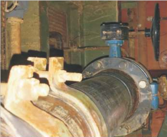
FEP Lined Butterfly valve in Steel company Acid line
